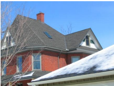
IDENTIFY AREAS PRONE TO ICE DAM FORMATION
