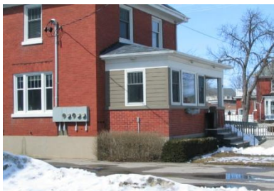
UTILITY METERS LOCATED ON A SIDE WALL
