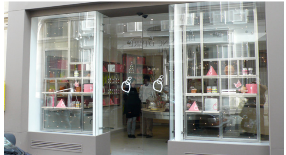
Barrier-free access and weather protection can be accomplished using recessed entries Paris, France
